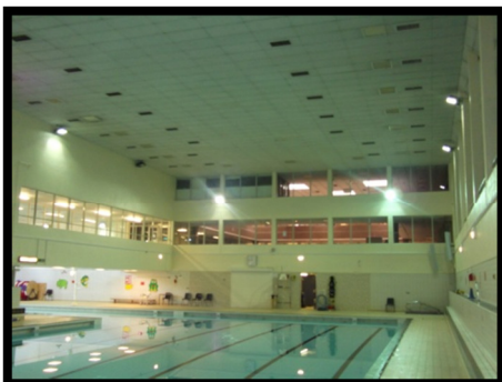
Before – Original suspended ceiling
